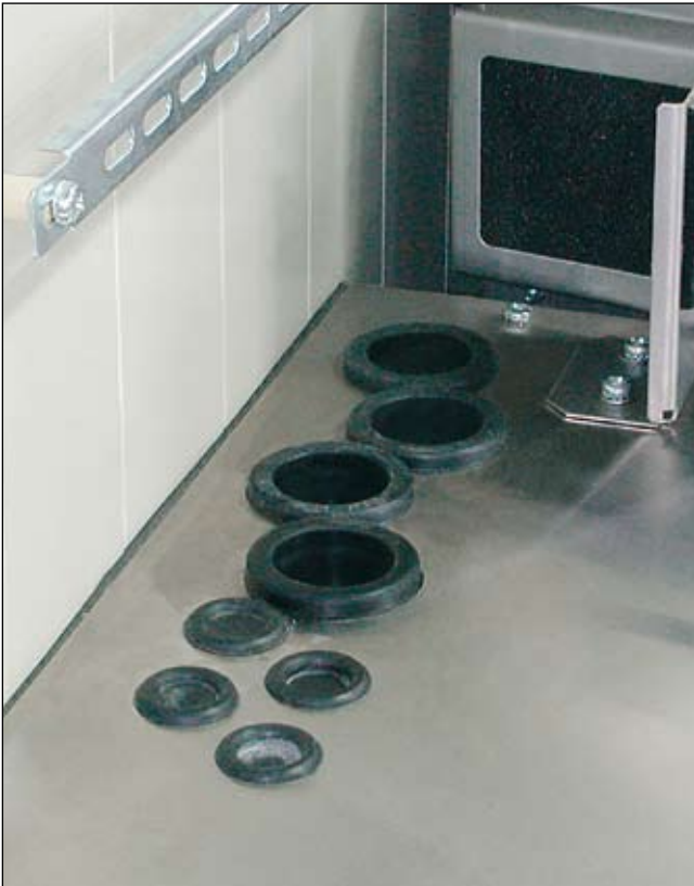
Cable entry made of rubber gland seals
