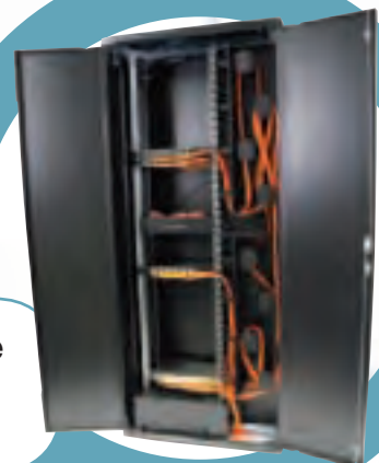
High Density Fibre Cabling Cabinet page 22
